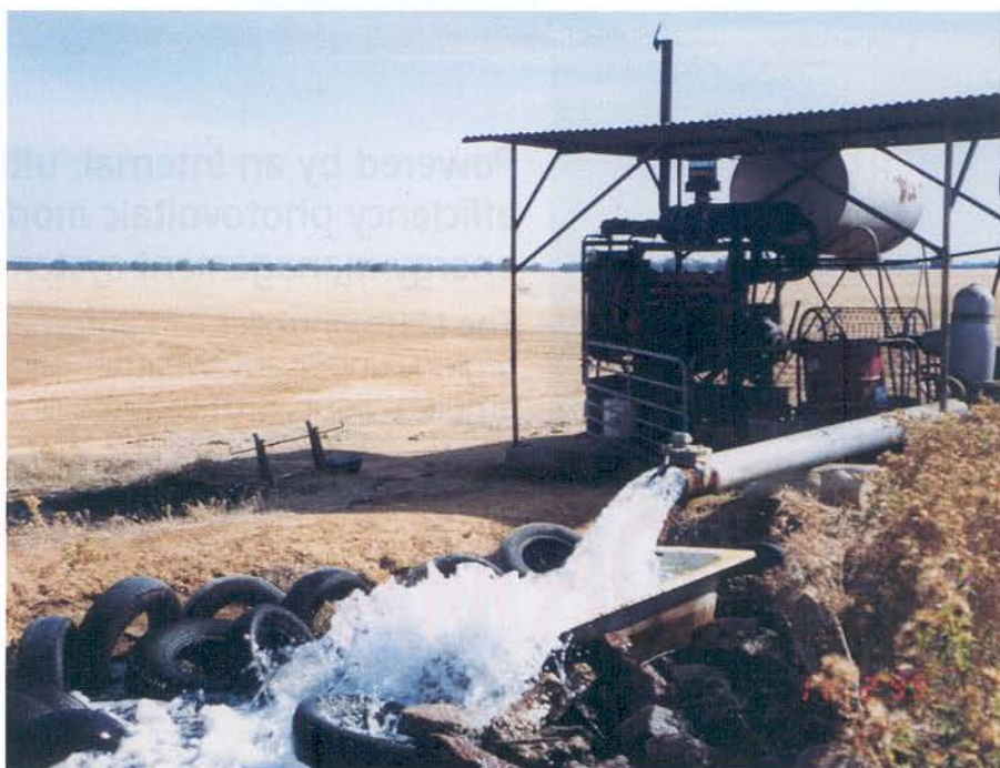
A typical deep irrigation bore, driven by diesel turbine pump
